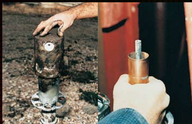
Burned PTFE shows the conductive path formed by dust-laden moisture. As the path arcs over, the transmission line fails.
